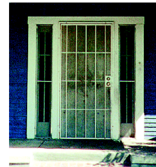
Inappropriate screen door
