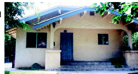
Inappropriate use of stucco over wood
