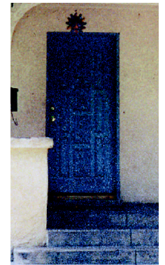
Inappropriate hollow core door
